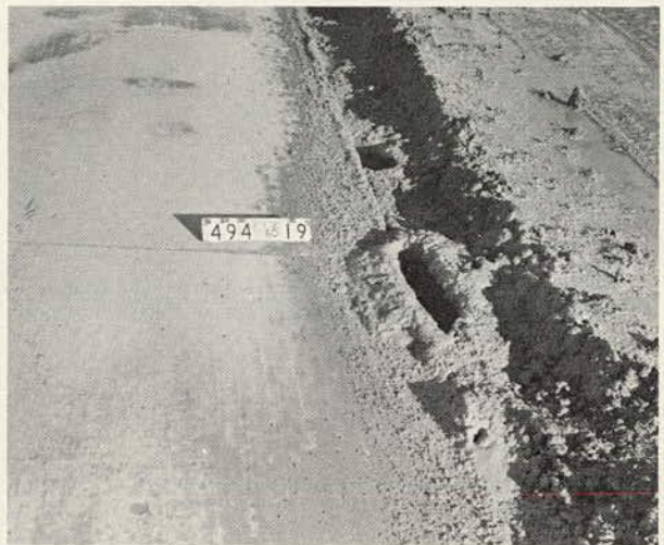
Embankment material pumped from beneath a pavement constructed without a subbase.
