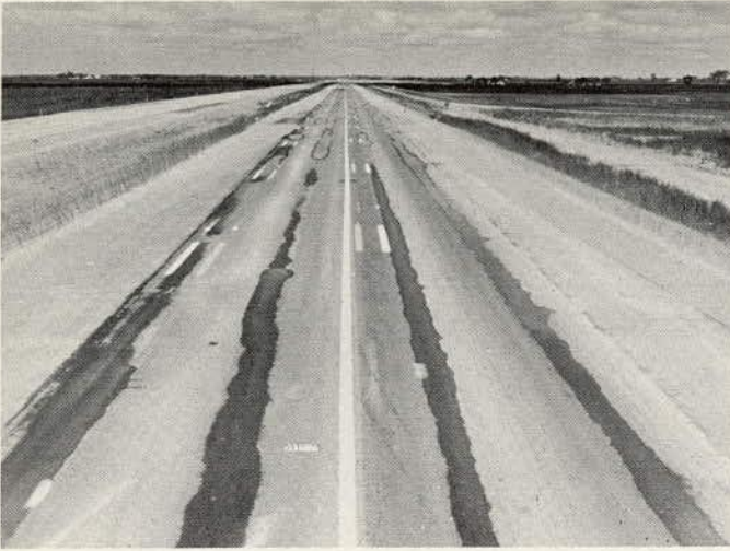
Evidence of longitudinal rutting, water in wheelpaths after a rain in a no-traffic period.
