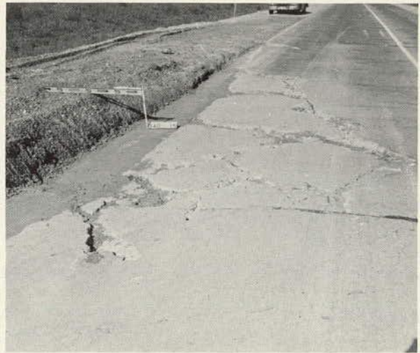
Subbase material ejected from beneath pavement overnight and deposited along edge.
