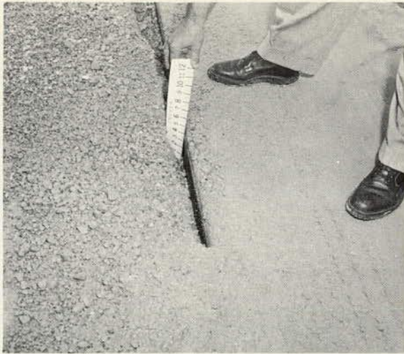
Void in shoulder through which subbase material was ejected from beneath pumping slab.
