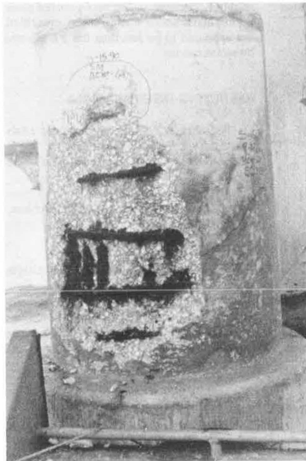
Figure 1 Typical corrosion deterioration common to Seven Mile Bridge observed in 1987.
