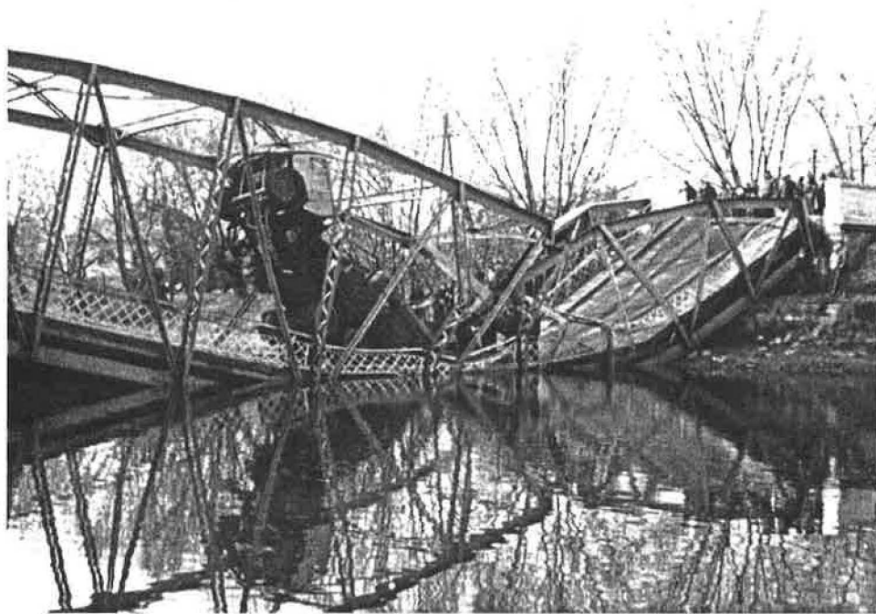
Figure 5: The bridge over Hernád at Gesztely deteriorated by the crash of an oversized vehicle.
