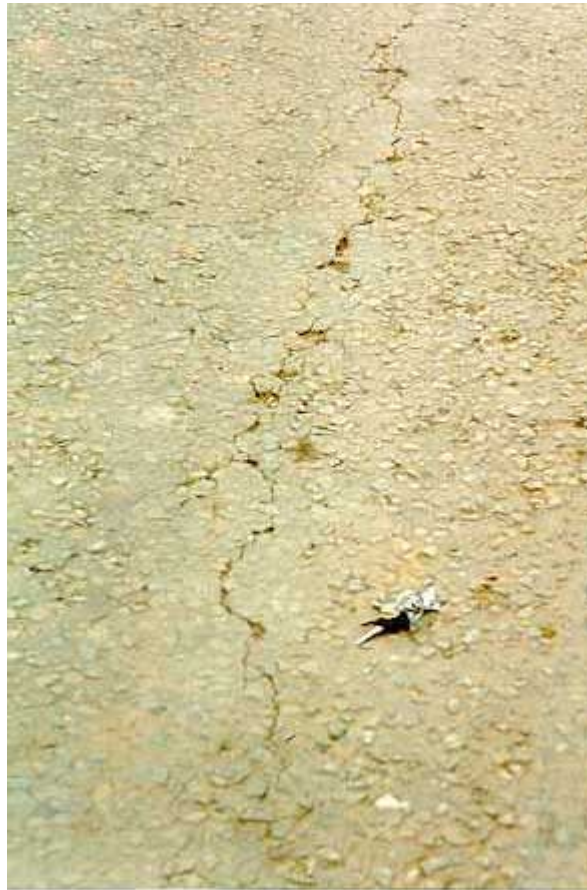
FIGURE 3a Longitudinal cracking in the near-side wheelpath of the M1 site.
