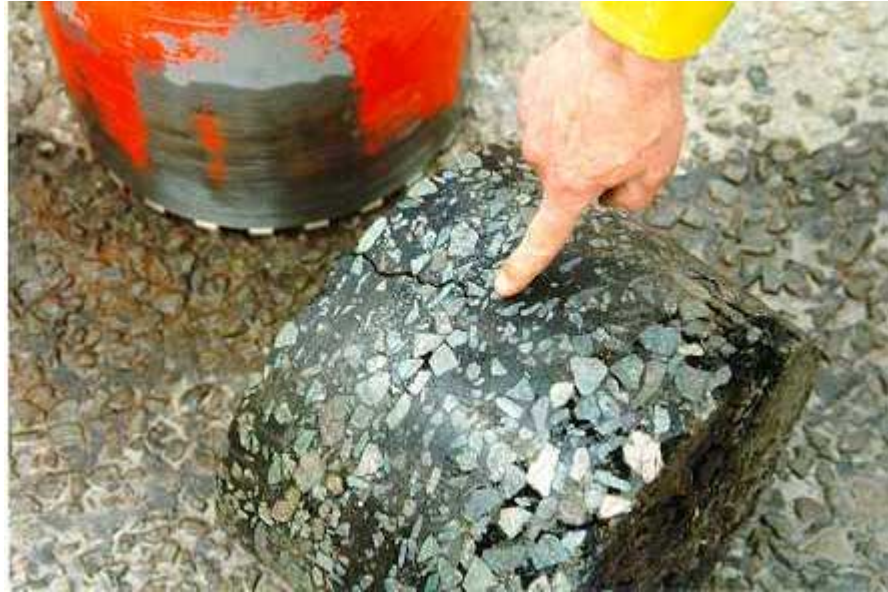
FIGURE 3b Longitudinal cracking in the near-side wheelpath of the M1 site.
