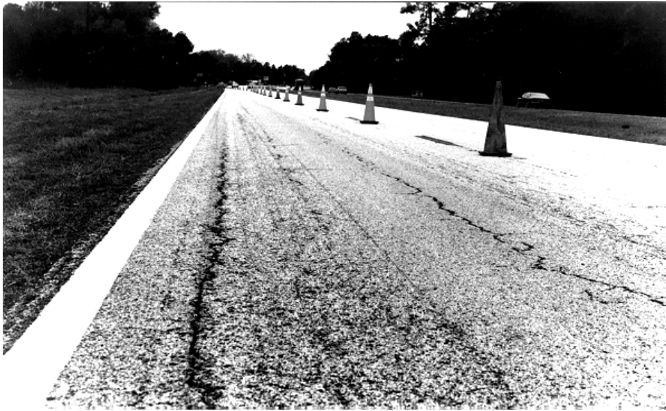
FIGURE 1 Lane exhibiting surface-initiated longitudinal cracks in both wheelpaths.
