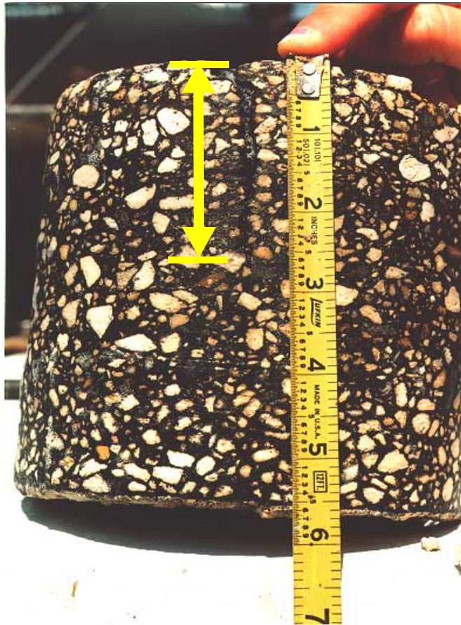
FIGURE 2 Core extracted from wheelpath illustrates crack opening at surface.
