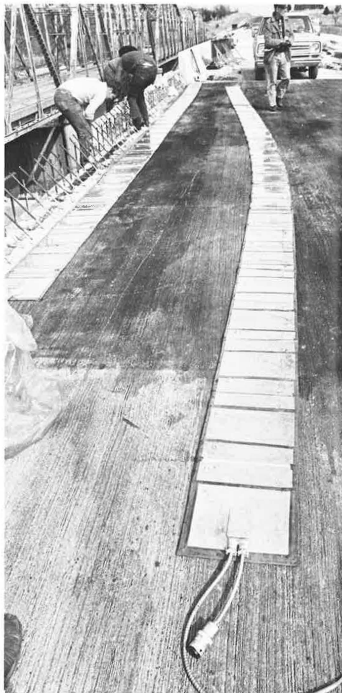
The electric blankets were made of stainless steel, contained a standard resistant type of heating element, and measured 38 cm wide and 14.6 m long. The old narrow truss bridge, which is being replaced by the present construction, is seen in the upper left corner.
