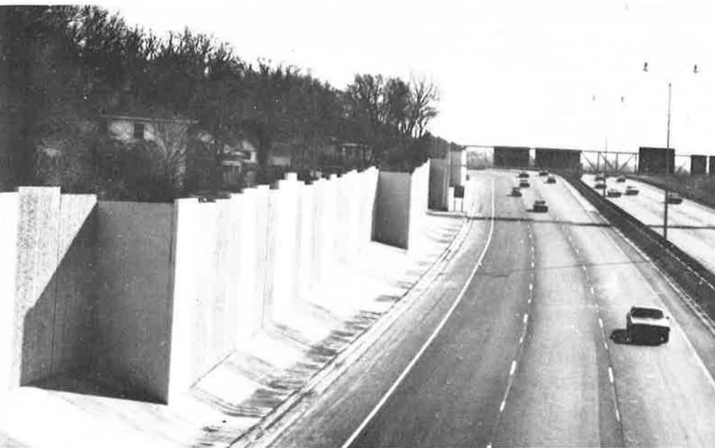
1 Air placing of concrete for experimental noise panels shows example of surface textures possible. When positioned above the noise path, walls like this have substantially cut decibel levels.
