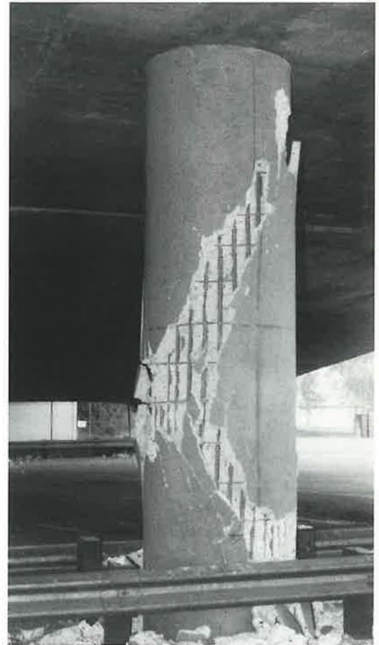
Column shear failure was one of several problems experienced by bridges as a result of the Northridge, California, earthquake of 1994.
