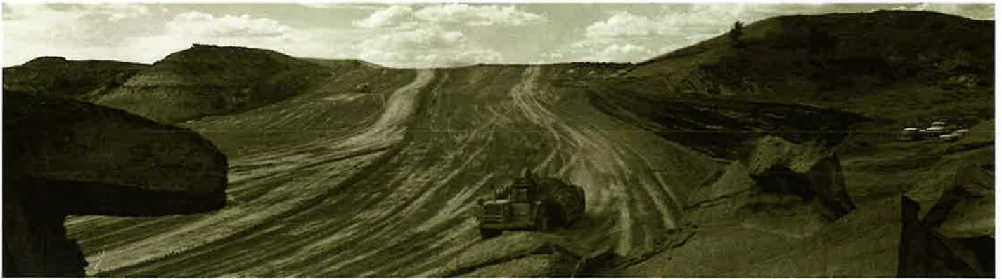
Path is cleared for construction on portion of Interstate 94 in North Dakota.
