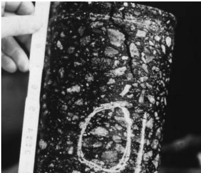
Core sample from I-287, showing top-down cracking.
