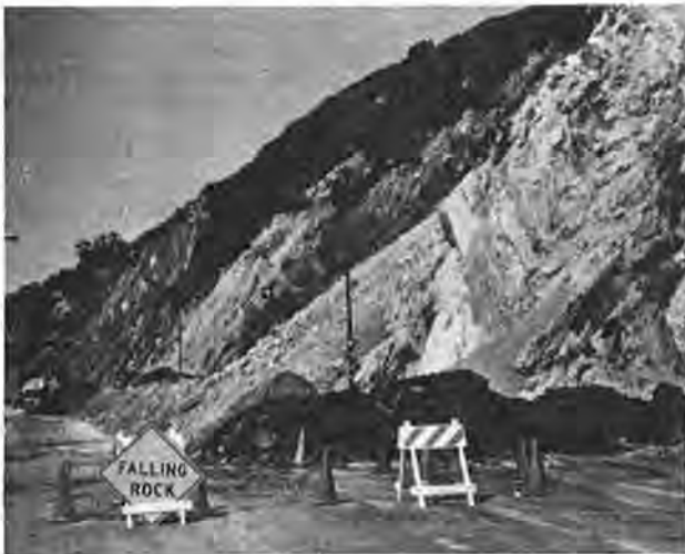
Figure 9. Soil berm catchment system on Pacific Coast Highway.
