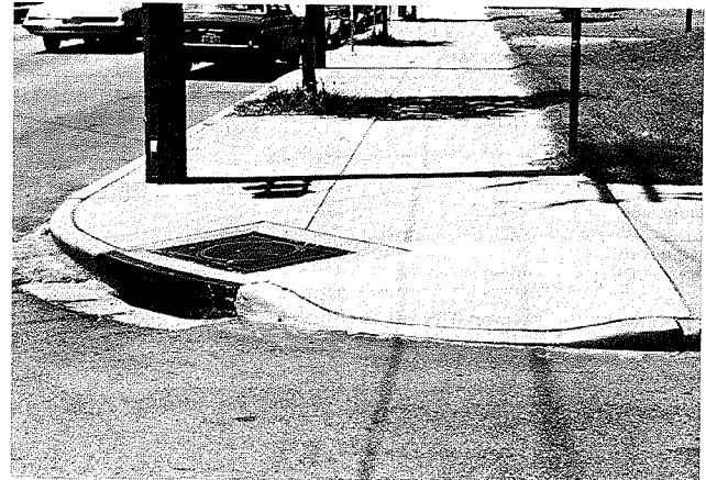
Figure 3. Curb ramp problem: drainage structure affecting placement.
