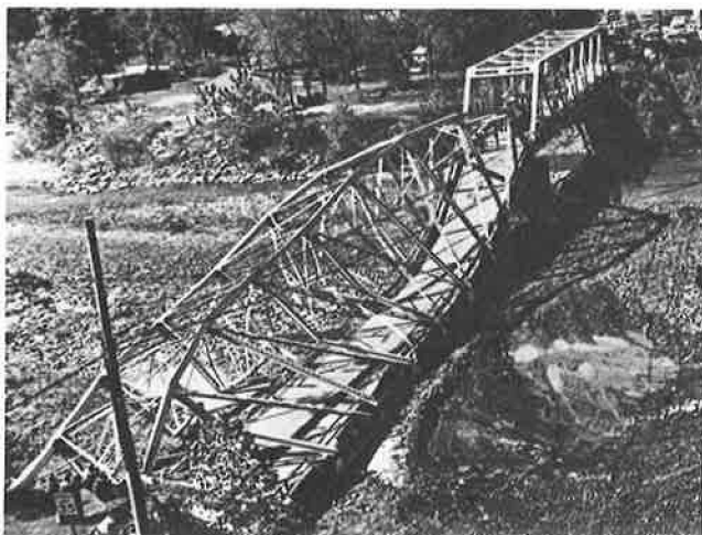
Figure 1. Through truss failure.
