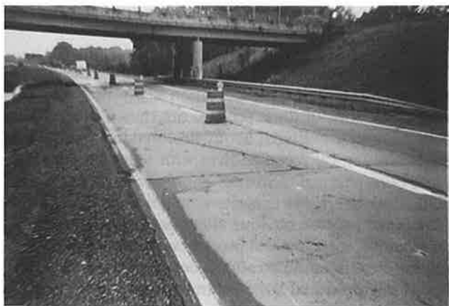
FIGURE 4 Deteriorated pavement section.
