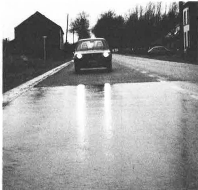
FIGURE 3 Difference in reflection of the headlights of a car on a wet road surface. In front, dense asphalt; behind, porous asphalt.
