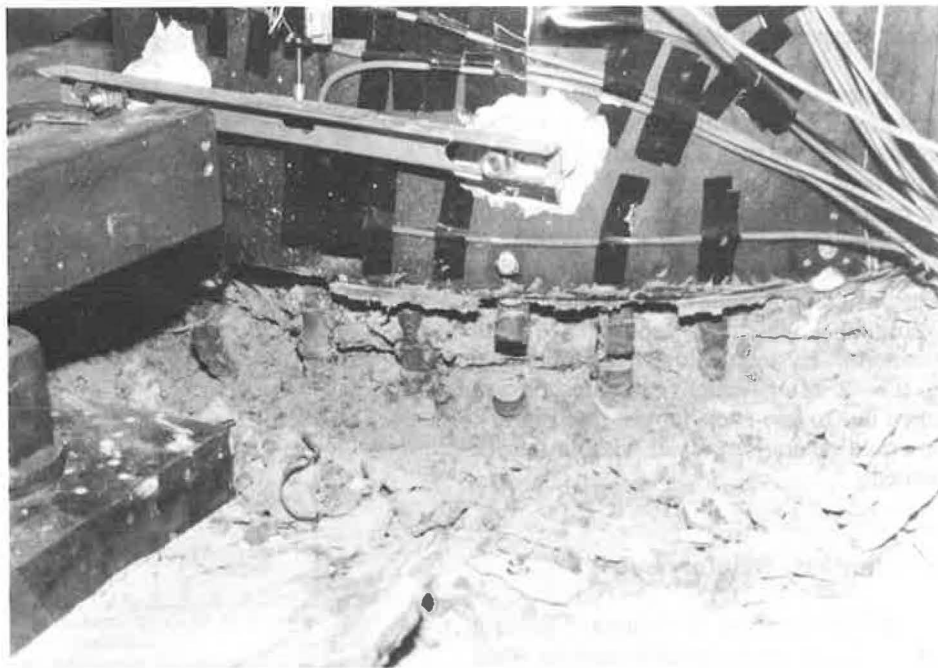
Figure 11: Low-cycle Fatigue Fracture of Main Steel in Column 6
