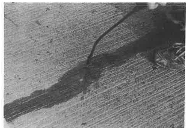
FIGURE 1 HMWM monomer applied to cracks in tined bridge. To maintain good skid number, excess resin in valleys must be broomed over deck surface before it gels.
