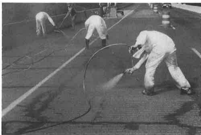
FIGURE 2 Airless spray guns were used to apply HMWM resin to surface of tined bridge deck. Note that work crew is wearing rubber boots and gloves, impermeable coveralls, and canister breathing masks.
