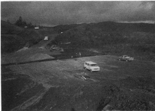
FIGURE 7 Wood fiber fill construction: top , granular fill construction and culvert installation; bottom , placement of geotextile and wood fiber fill.
