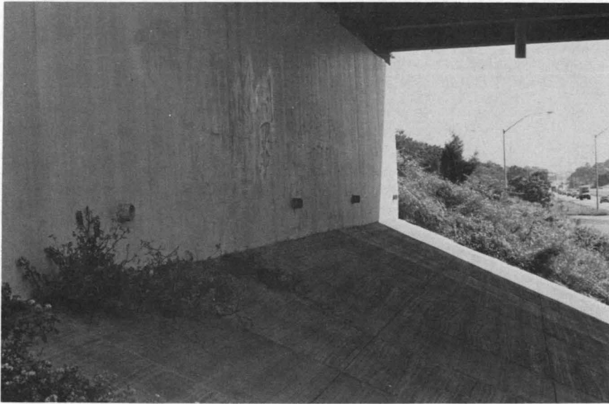
FIGURE 2 Short vertical metal pipe that spills directly onto abutment slope.
