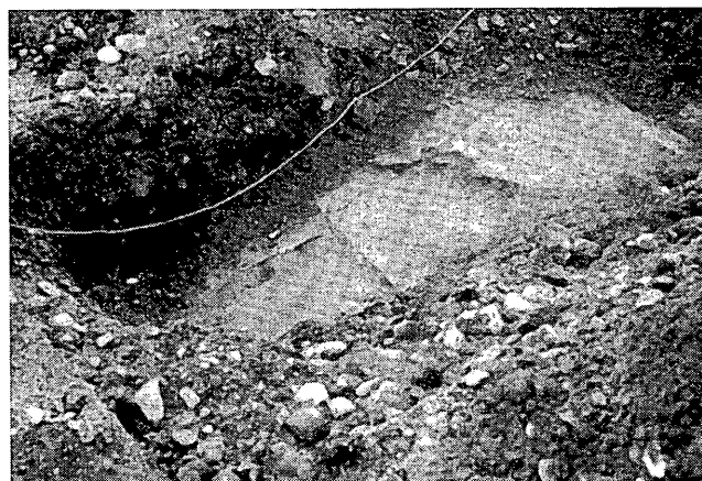
FIGURE 6 Damaged and overlapping insulation panels, Station 30+00, Newton Field runway.
