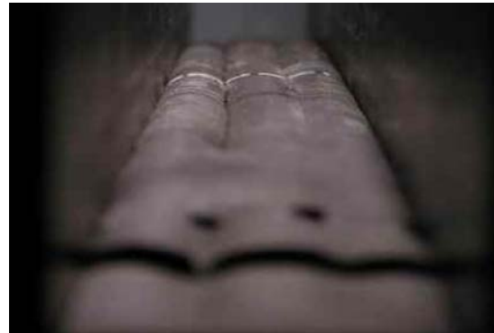
Figure 2.2 Initial Debonding of Bearing
