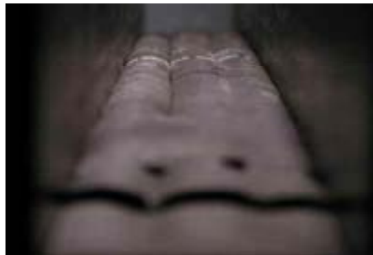
Figure D-15. Debonding Visible at Surface of Bearing
