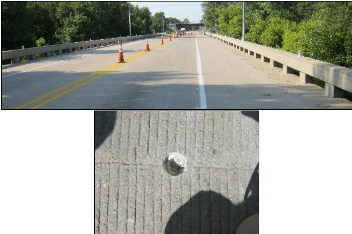
FIGURE 29 (Top) photograph of Nebraska Bridge Deck 1 on which scanning took place in the southbound lane and shoulder and (bottom) photograph of a chloride concentration sampling location that corresponded to a construction joint characterized by lower impedance values.
