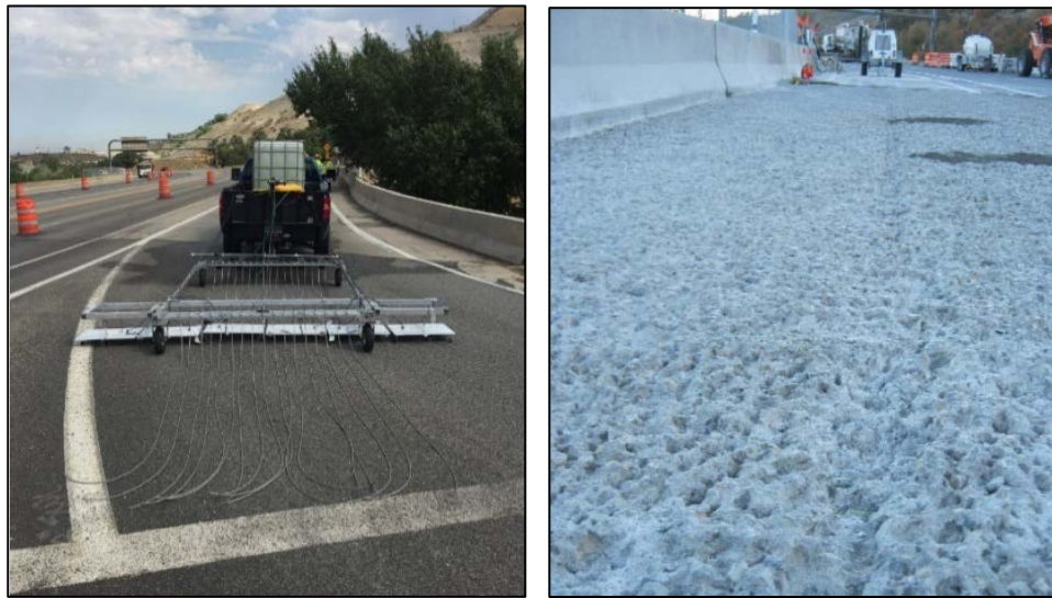
FIGURE 25 (Left) impedance testing of an outer lane on a bridge deck with a PPC overlay in northern Utah and (right) scarified surface of the same bridge deck prior to application of the PPC overlay.
