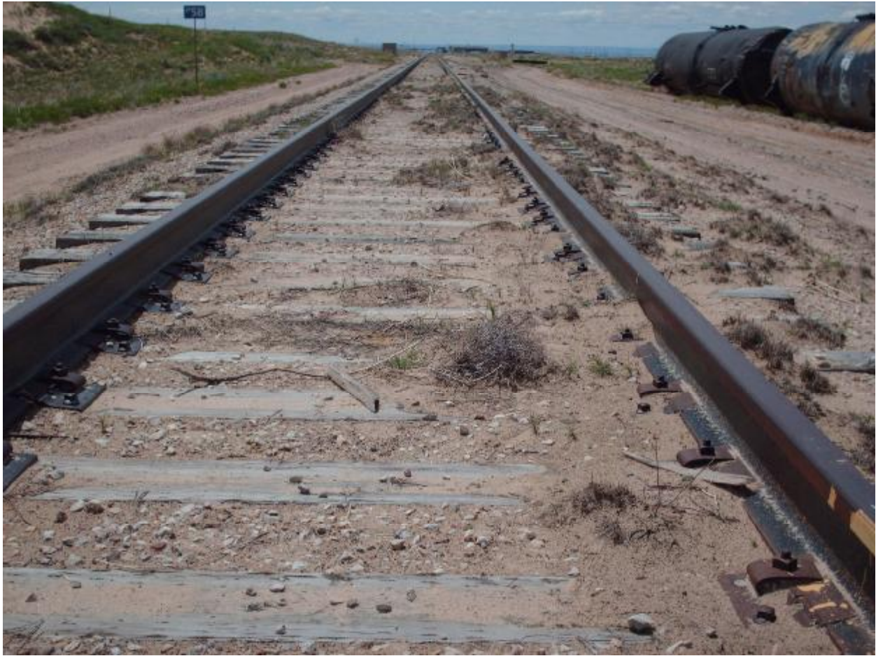
FIGURE 4 PTT Picture of Dirt and Dust Build-up in Ballast.
