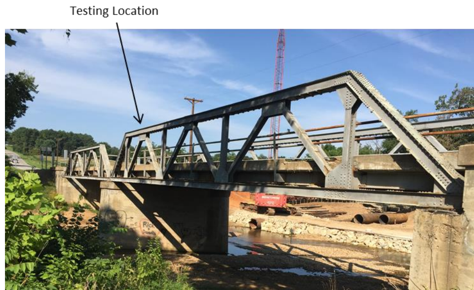
Figure 21. Side view photograph of the pony truss bridge used for field testing.
