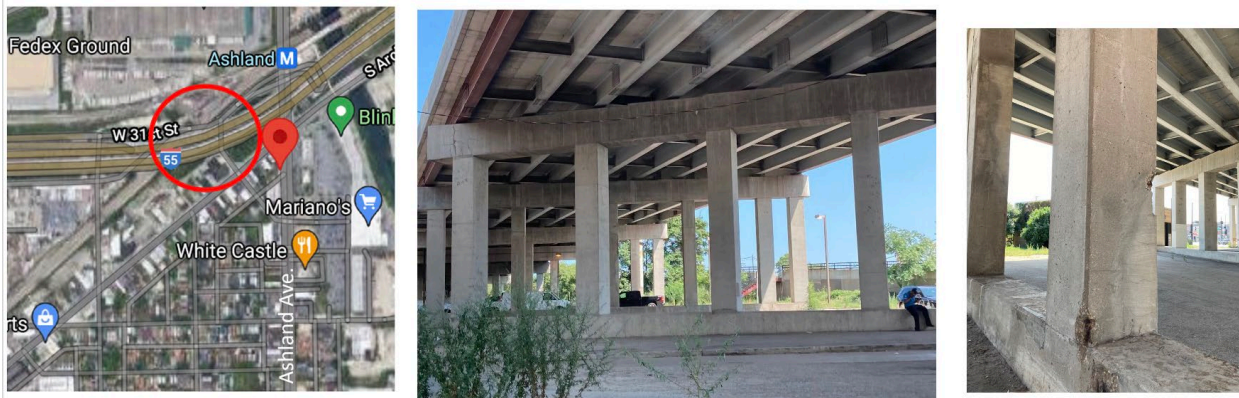
FIGURE 21 The location of bridge pier under I-55 (left), a photo of bridge piers (middle) and a photo of the bridge pier measurements taken (right).
