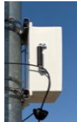
Figure 4 External Battery for 7 Days Operation
