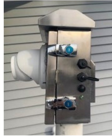
FIGURE 3 System Interface on the Side of the Box
