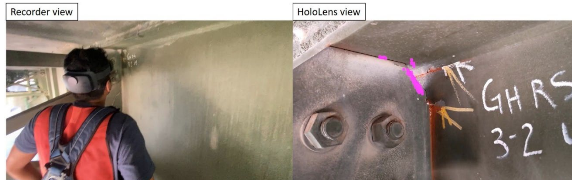
Figure 88 Inspecting the detected crack area with threshold value of 0.38
