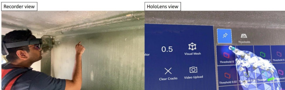
Figure 83 Hitting the button with zero threshold value to see the whole region analyzed for crack detection
