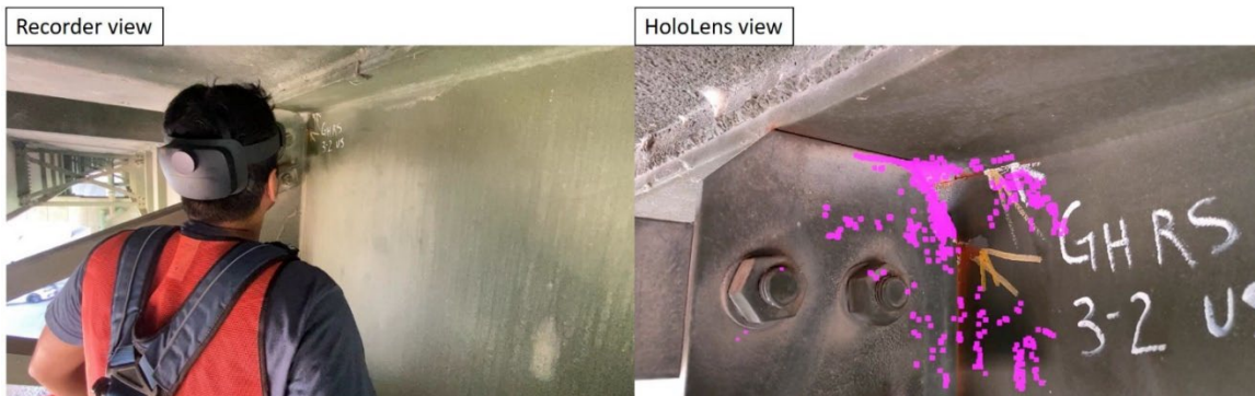
Figure 86 Inspecting the crack detection result for threshold value of 0.2
