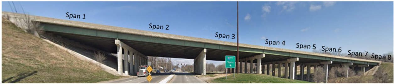
Figure 72 Span layout of the I-70 highway bridge with Span 3 selected for testing
