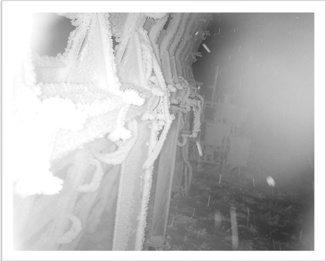
FIGURE 26: Freezing drizzle accumulating on the underside of the solar snow fence.
