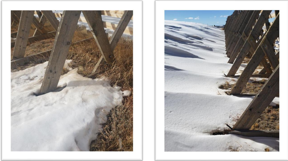
FIGURE 18: Snowdrift creep and glide onto the existing wooden snow fence at the test site.
