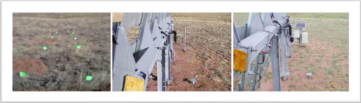
FIGURE 28: Native vegetation prior to the start of construction (left – photo taken first week of November 2021); area around the solar snow fence immediately after construction (middle – photo taken the second week of November 2021); and revegetation without reseeding (right – photo taken in June 2022).
