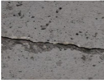
Figure 4-1 Example of a concrete crack on a bridge.
