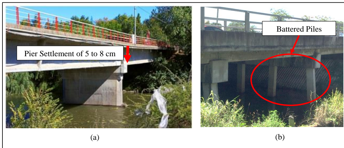
Figure 2-1 Examples of (a) bridge settlement and (b) battered piles.
