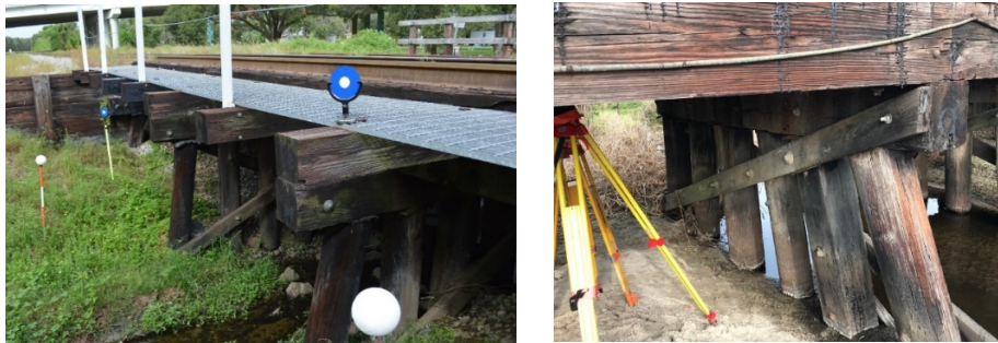
FIGURE 27. As-is condition of the open deck bridge in Valrico; As-is condition of the ballasted-deck bridge in Lorida
