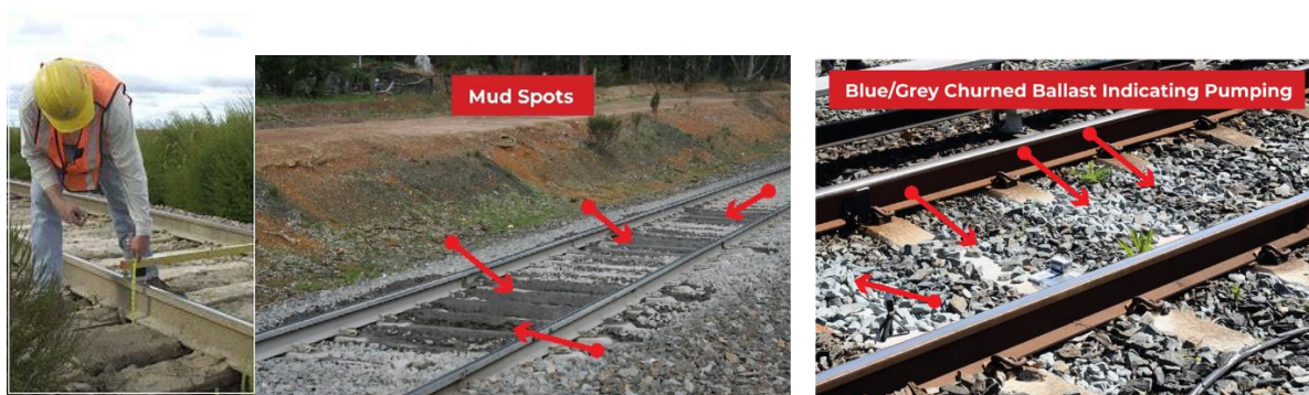
Figure 5: Track Inspector inspecting key problem areas such as Mud Spots and signs of pumping
