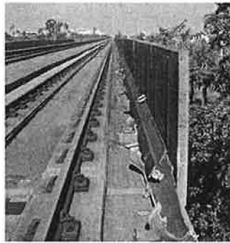
Cover board blown off along with third rail during Hurricane Wilma, Miami, October 2005
