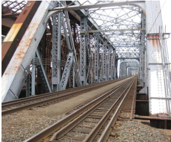
Figure 1: Span 7 of the Devon railroad bridge showing the open deck floor system and the truss structure.
