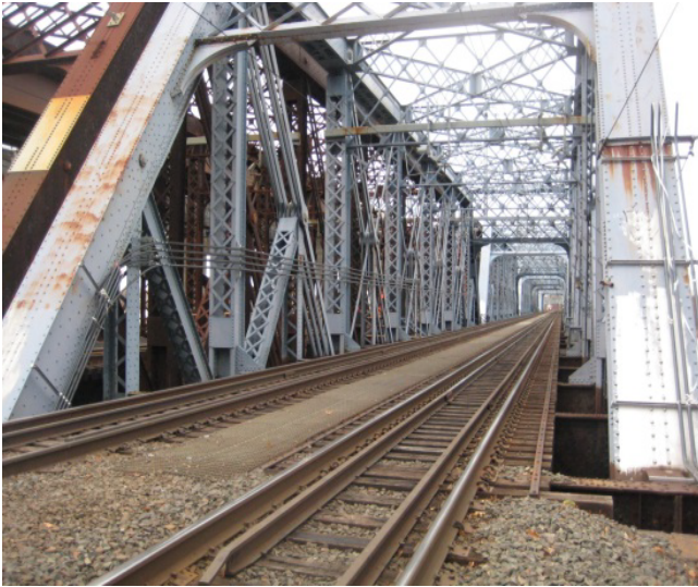
Figure 1: Span 7 of the Devon railroad bridge showing the open deck floor system and the truss structure.
