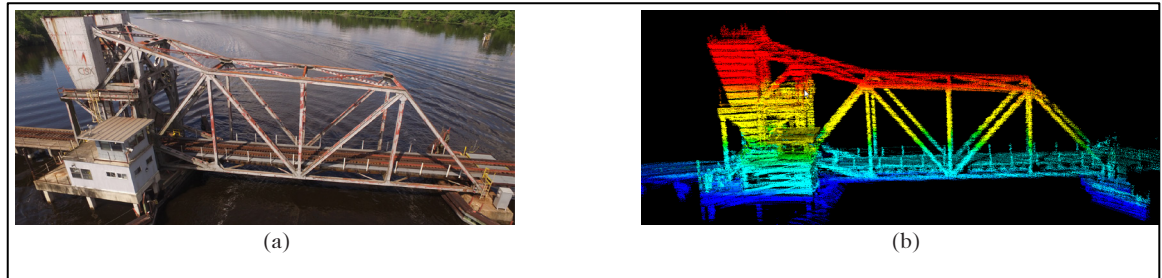
Figure 3: (a) CSX's railroad drawbridge; (b) 3D model of drawbridge from LiDAR data.
