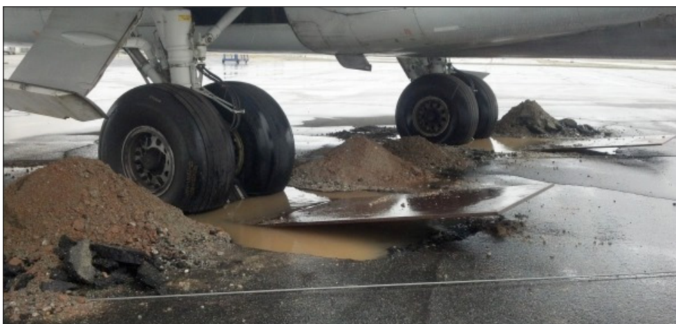
Above: A disabled B727 aircraft is parked on steel plates during its recovery process on the ramp at KRAL airport in Riverside, CA. Following the recovery, permanent concrete pads were poured for long-term parking of the aircraft at KRAL, and asphalt repairs were made to return the ramp to normal use. Image courtesy of C. Daniel Prather, Ph.D., CBU.
