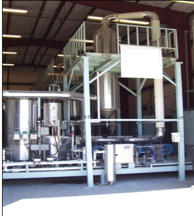
Figure 2. MVR unit at Denver International Airport (courtesy of Inland Technologies).
