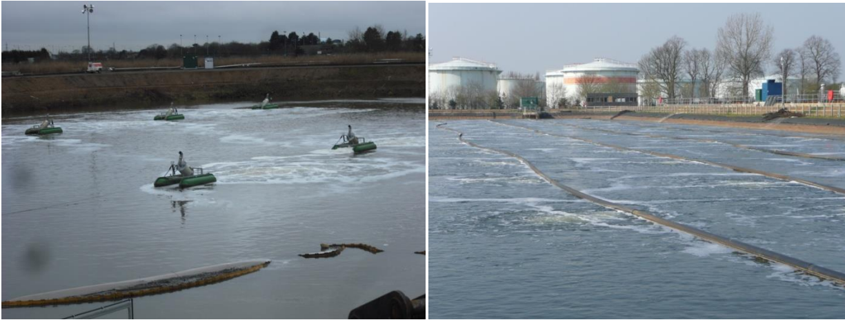
Figure 2. Aerated lagoons with aspirators (left) and submerged diffusers (right) (courtesy of Mark Liner).
