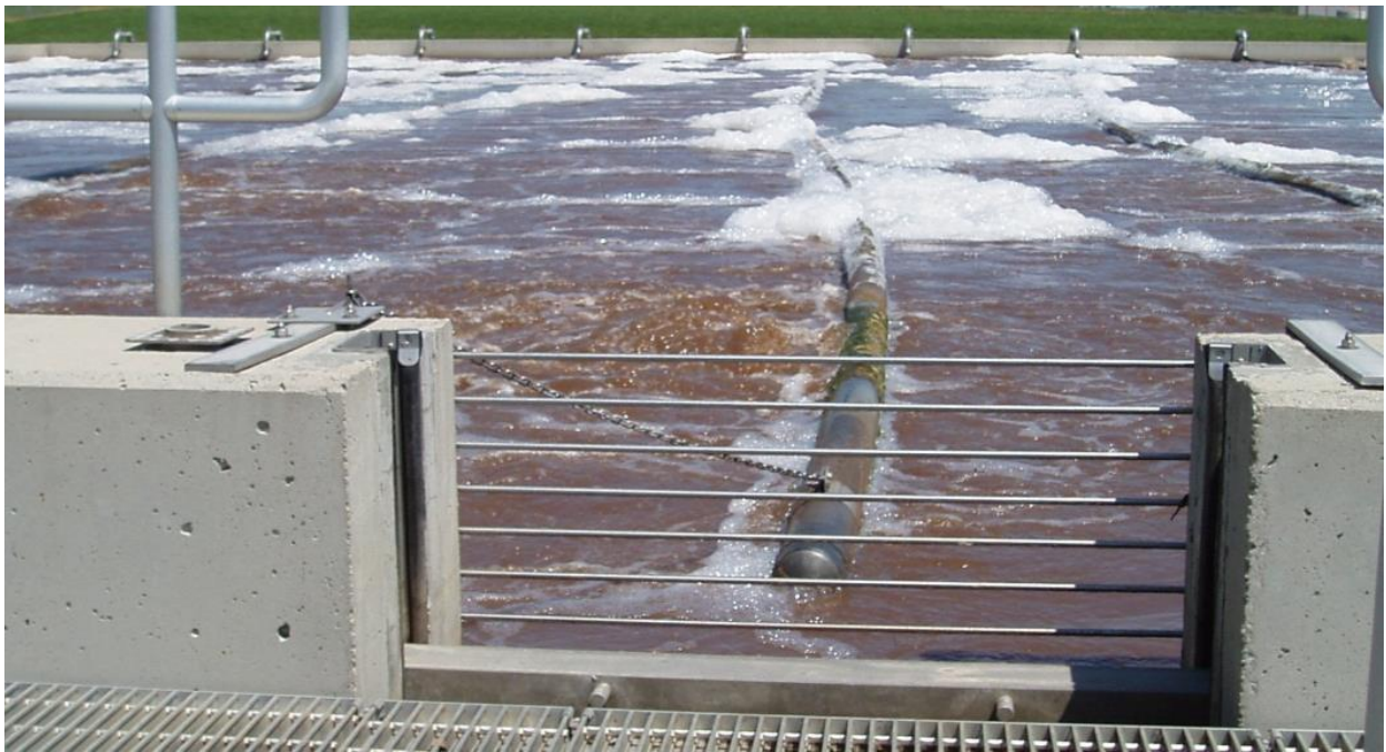
Figure 2: Activated sludge aeration basin (courtesy CVG Airport).
