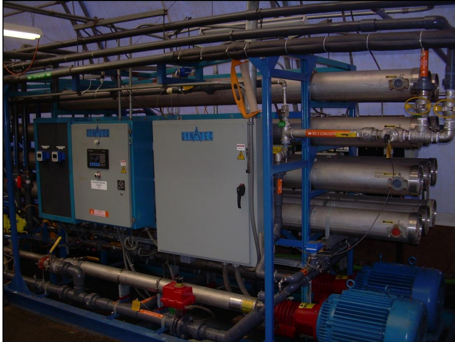
Figure 2. RO system at Bradley International Airport.
