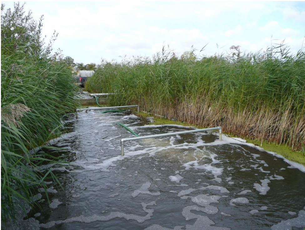
Figure 5. Partial mix aerated channel (courtesy of ARM Group LTD).
