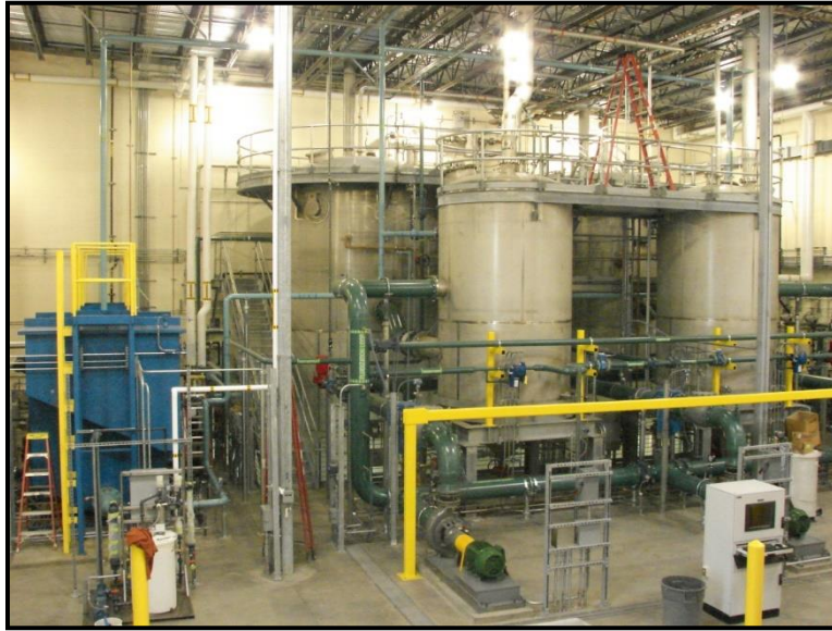
Figure 3. Reactor units in the PDX AFBR system.
