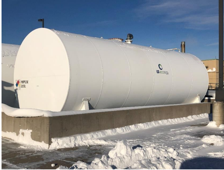
Figure 3. Concentrate storage at the glycol management facility.
