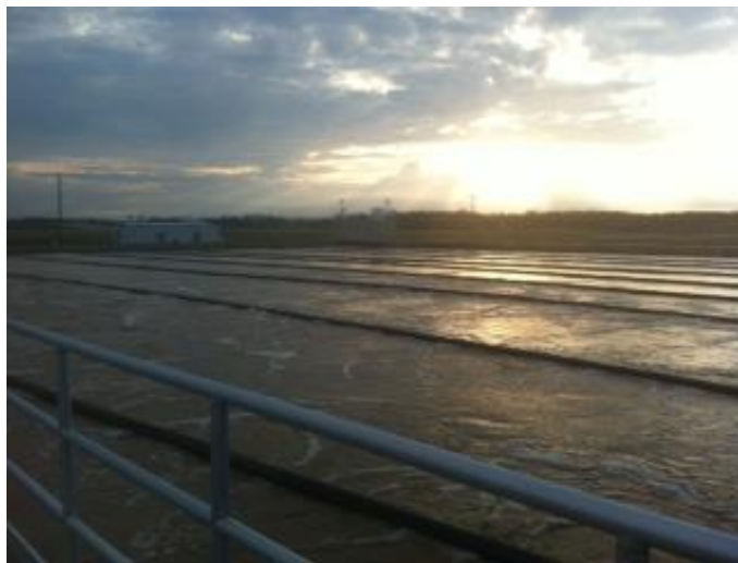
Figure 3. CVG's activated sludge treatment system aeration basins.
