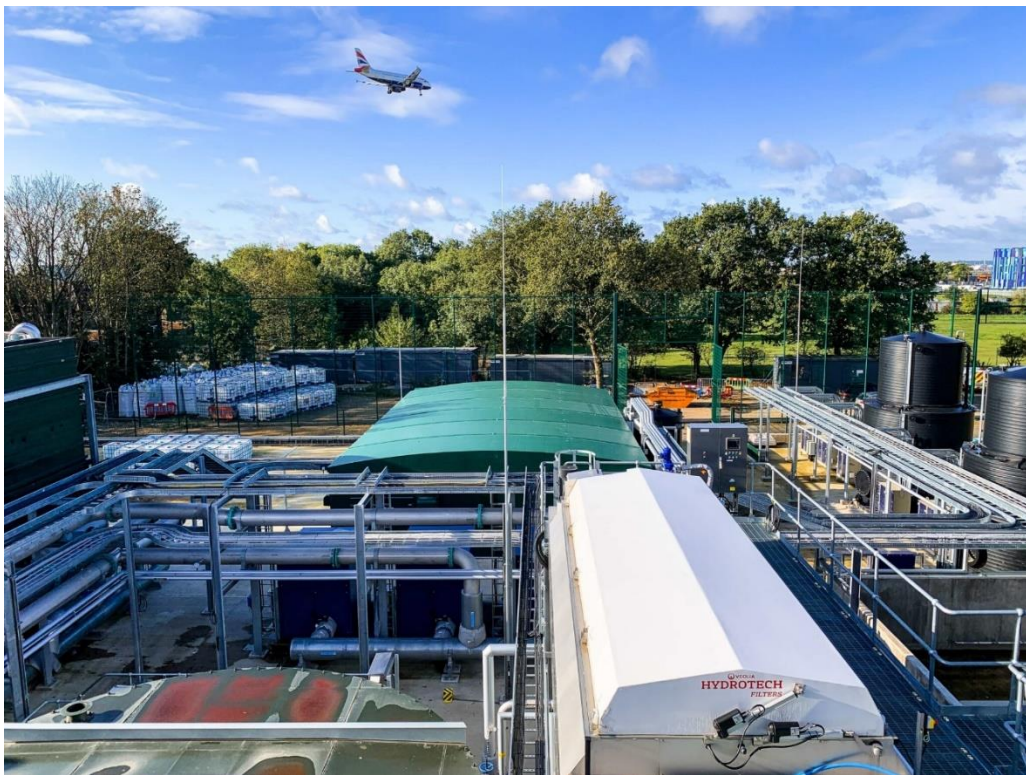
Figure 5. Disc filter and piping (Enviropro, 2022).
