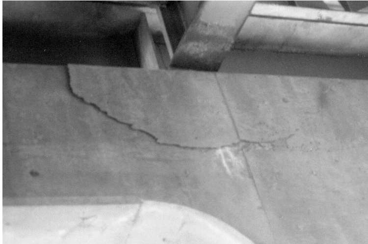
Figure 1. Photograph of Typical Damage Caused by Inadequate Allowances for Bridge Movement
