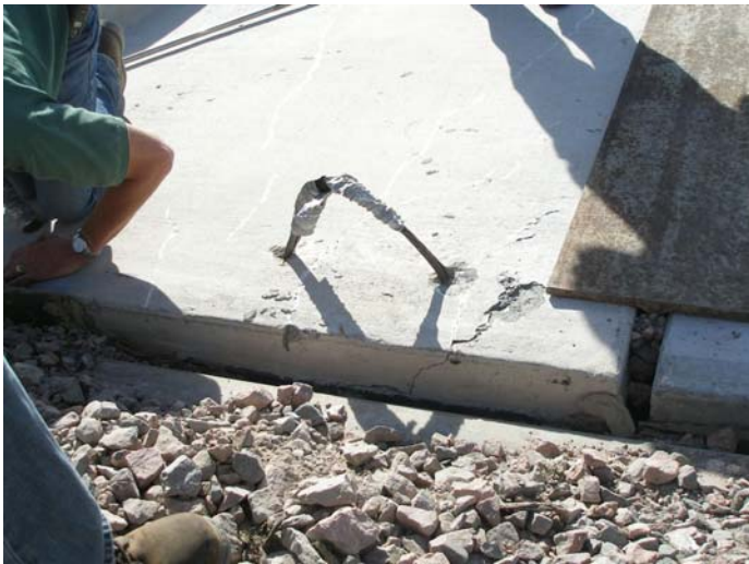
FIGURE 4.12 Shear Cracks in Overlay – Post Test
