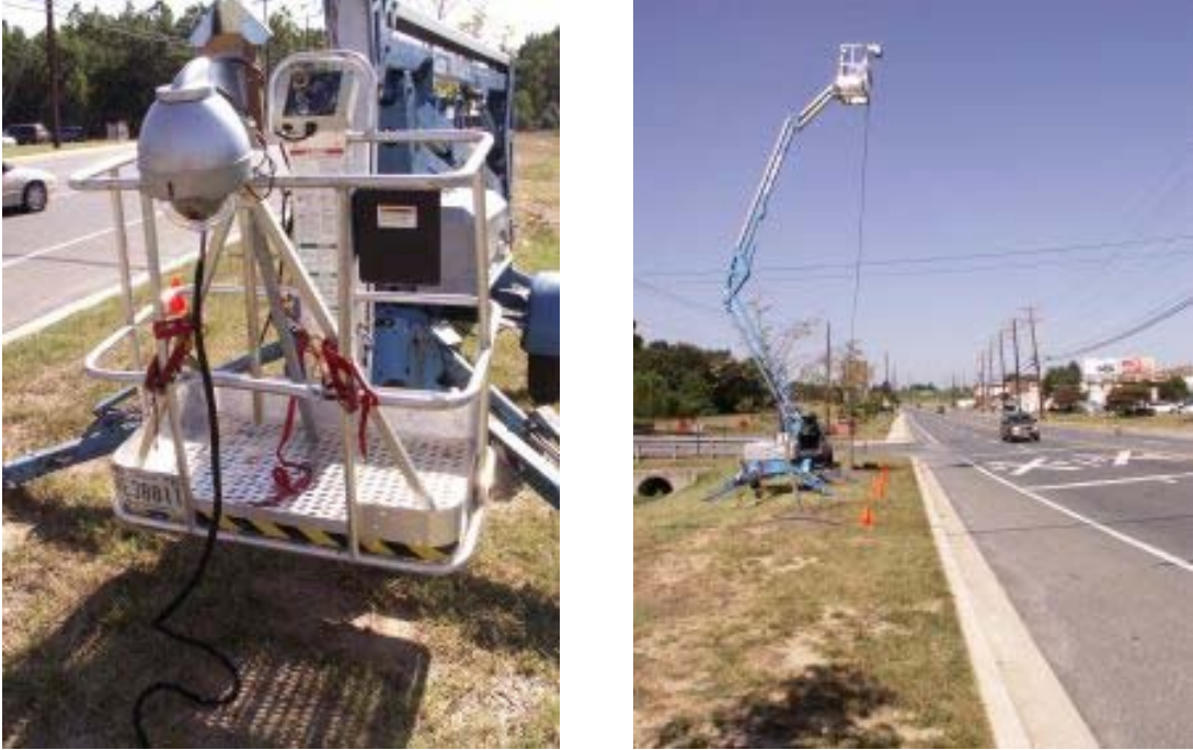
FIGURE 11. Aerial lift with camera, shown with lift arm retracted (left) and extended (right)
