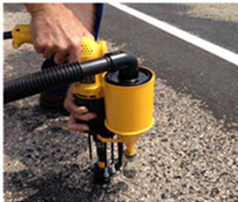
FIGURE 3 Homemade Venturi dust collection system.
