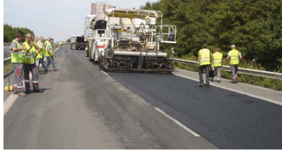
FIGURE 8 7,000 T of EME 0/20mm with 65% RAP on the French A26 toll highway near Arras.
