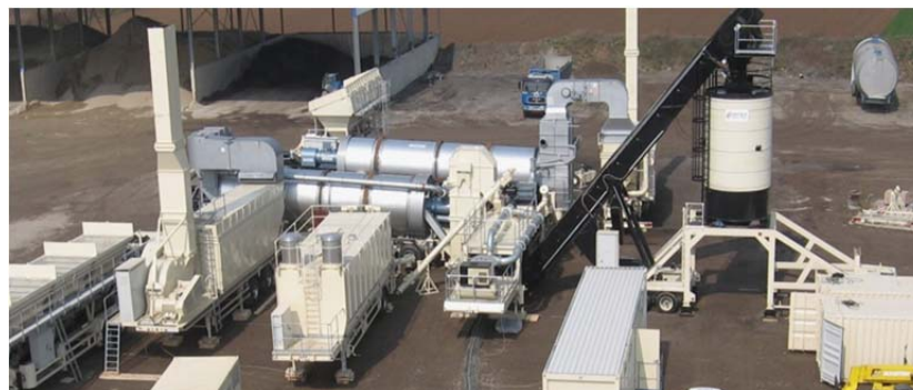
FIGURE 5 In-house mobile parallel drum plant of EIFFAGE TP group: (a) overall view and (b) view of the two parallel drum dryers (the first one for virgin aggregates, the second one for RAP).
