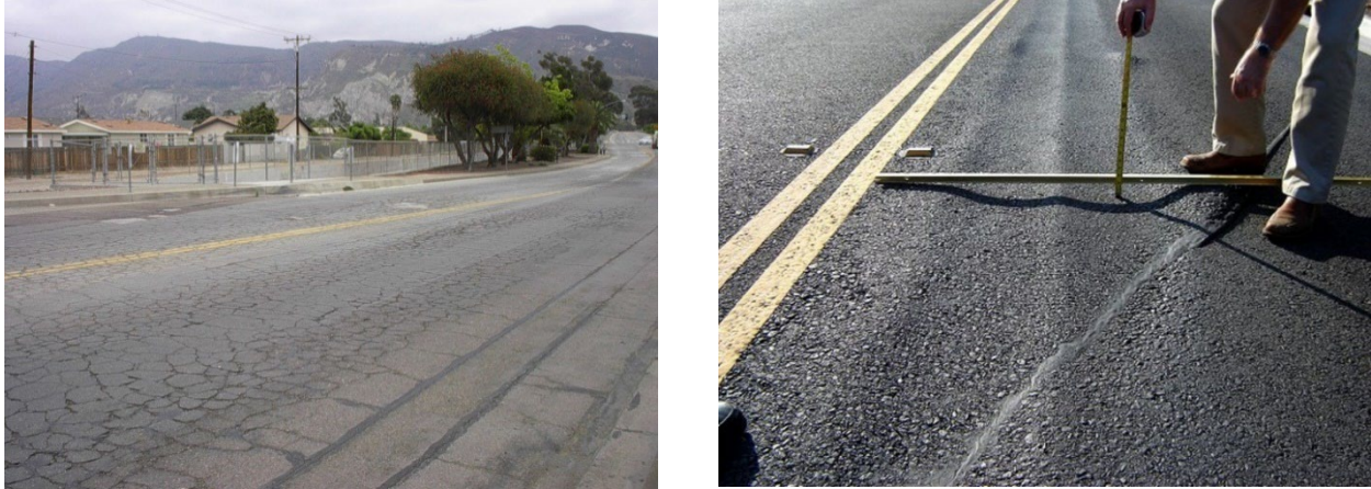
Figure 4.3 Load-related cracking (left) and rutting (right) on asphalt concrete roads. (Image credit: RoadResource.org.)
