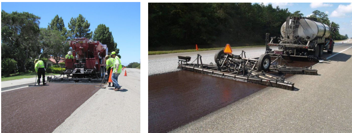
Figure 4.5 Application of a slurry seal (left) and scrub seal (right) on AC roads (image from RoadResource.org.)
