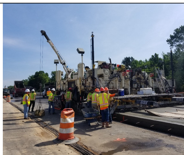
Figure 48 Mainline concrete pavement for I-85 PEM pilot project for concrete paving mixtures.
