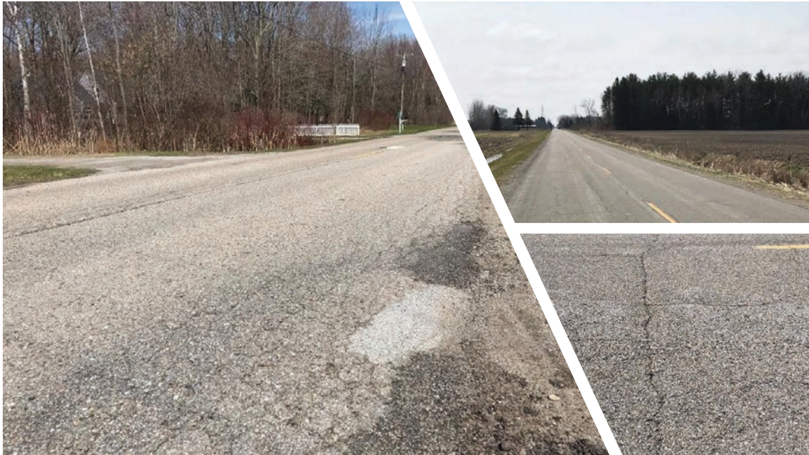
FIGURE 18 Pre-construction photos of some of the Michigan construction sites showing high levels of pavement distress.
