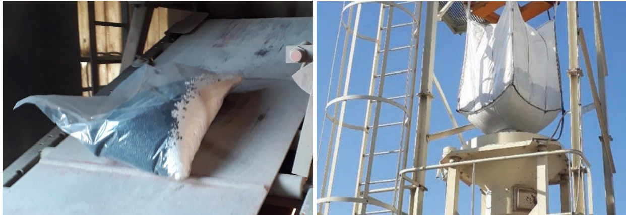
FIGURE 2 Addition of rPE at asphalt production facility: (a) rPE meltable bag introduced in a batch plant and (b) rPE big-bag dosed with hopper in continuous plant.
