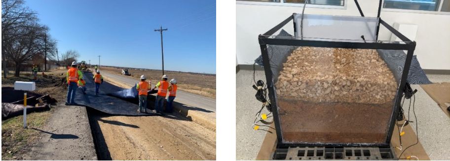
FIGURE 3 (a) Construction of test sections in Venus, TX, and (b) Laboratory test setup.
