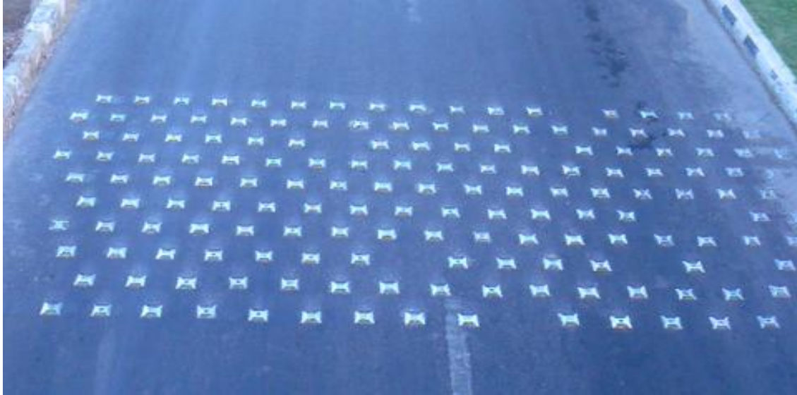
Figure 2 Sample to cat-eye reflectors at one site
