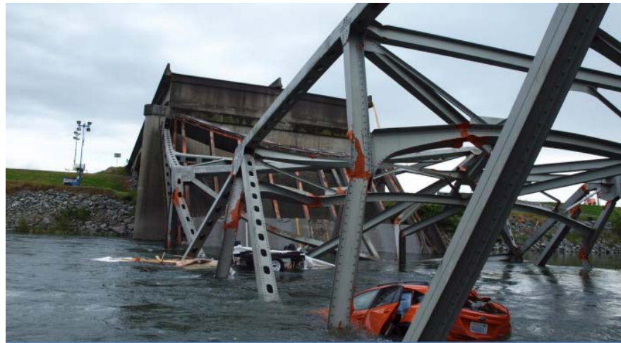
The Sufficiency Rating (SR) for the Skagit River Bridge was 53.8. Was that unsafe?
