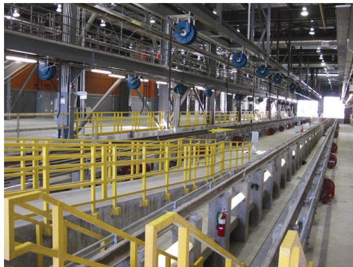
Metro East Operating and Maintenance Facility
